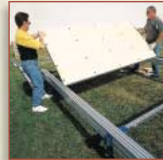
A small crew can set up the lightweight STRATA System in just hours.
