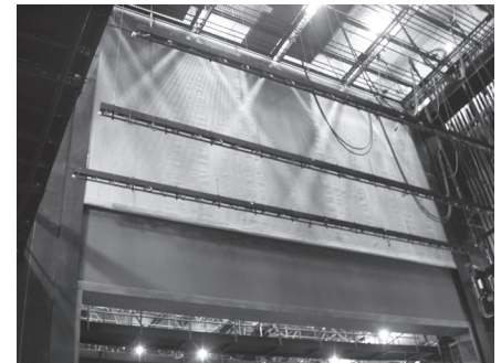
Straight Lift Fire Curtain
